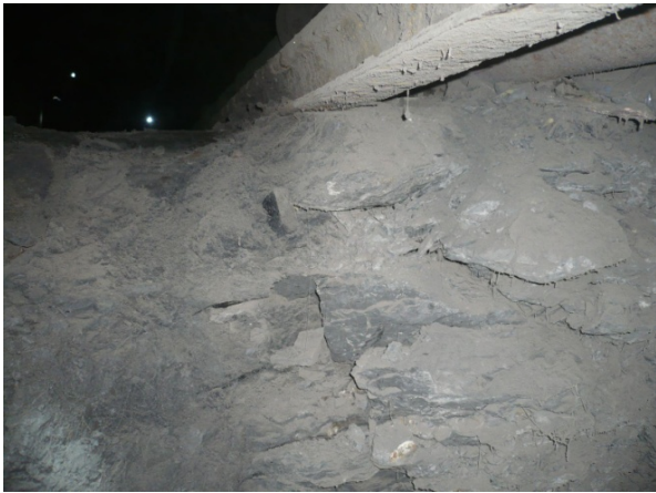
Figure 4. General view of floor rocks shear of a belt roadway of western longwall 12 of seam c_{18}
