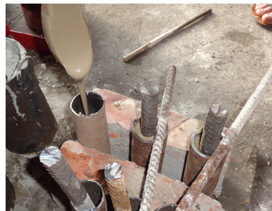
Figure 3. Mounting of anchor, fastened by means of a mixture extending while hardening, in the models simulating rocks: (a) with the help of concrete in a plastic form; (b) with the help of concrete in a metal form; (c) with the help of steel pipes
