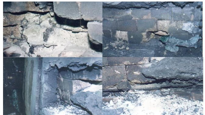
Figure 5. The damages of the refractory lining in the electric furnace No. 2
