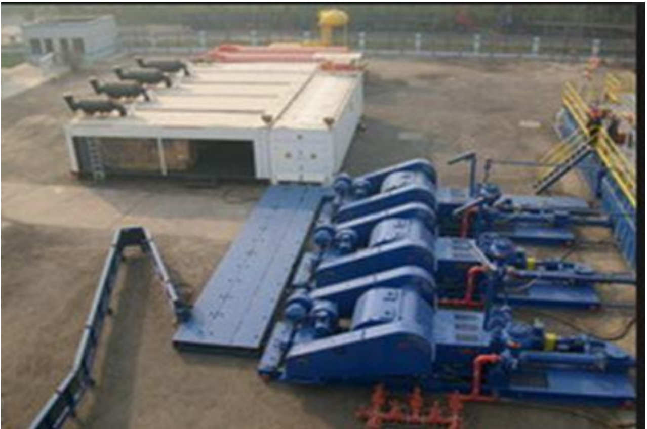
Figure 2.8 - Drilling Rig Power Generation System
