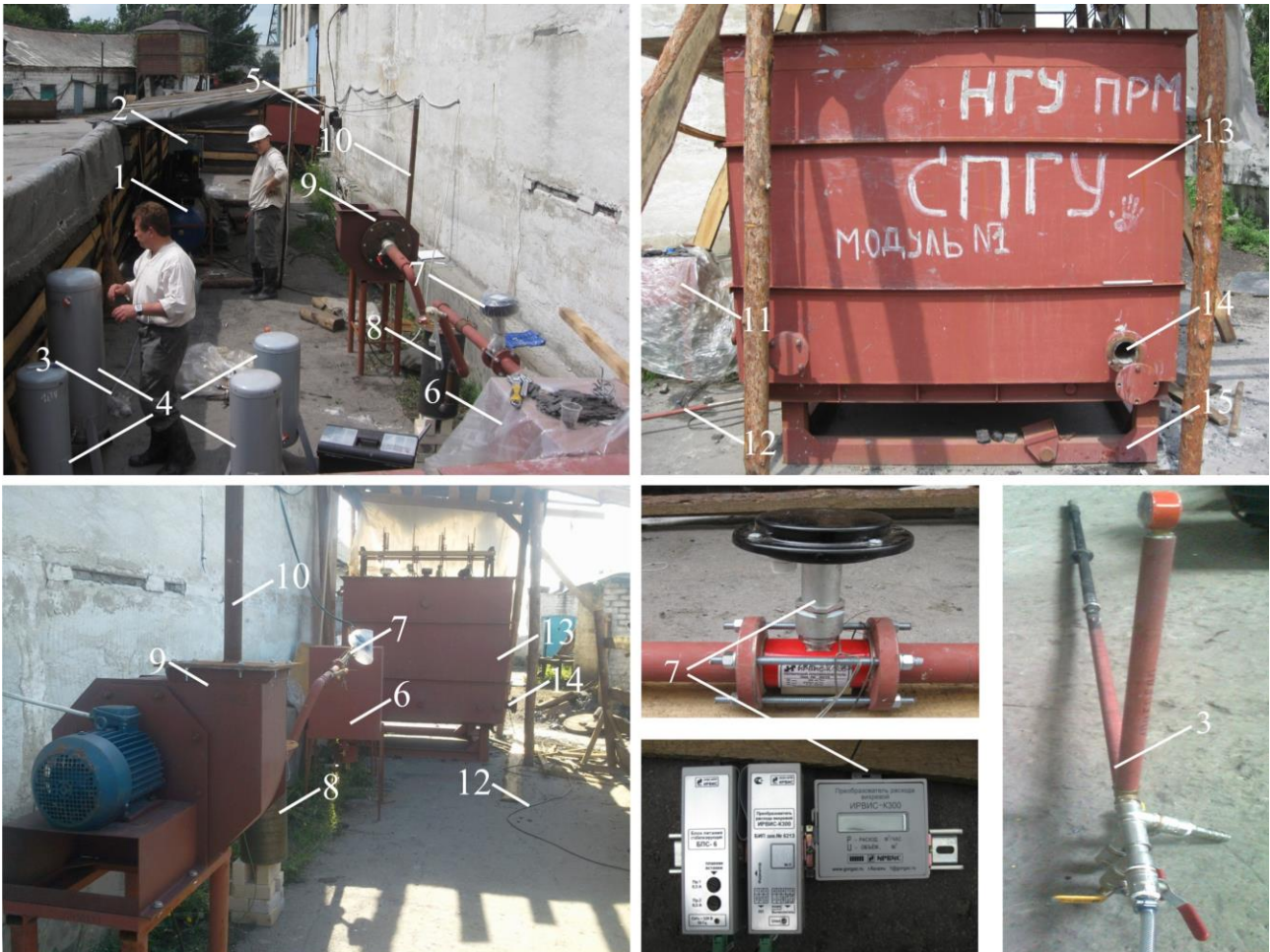
Fig. 1. General view of the operating systems: 1 – compressor RM-3138; 2 – steam generator AVPE-11/9; 3 –high-pressure pipeline; 4 – receiver (air, steam and oxygen ); 5 – a water reservoir; 6 – a tank-cooler; 7 – flowmeter IRVIS-300C; 8 – lime filter (catching of H 2 S); 9 – exhauster DR-1,0-00.00PS; 10 – offtake; 11 – tank of dew and slags collection; 12 – flexible pipeline; 13 – the stand setting; 14 – ignition borehole; 15 – platform for coal seam angle simulation
