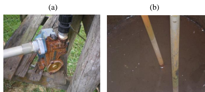
Figure 7. Rust formed on the iron pipe (a); rust formed on the galvanized pipes (b)
