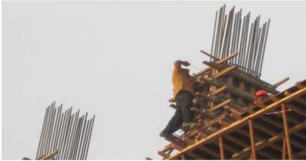
No Safety Belt used
